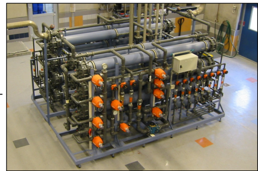
Swedish drinking water plant of 48 m 3 /h. The plant consists of 2 x NF 03-24, prefilter and fully automatic cleaning unit. Application: softening of ground water.
